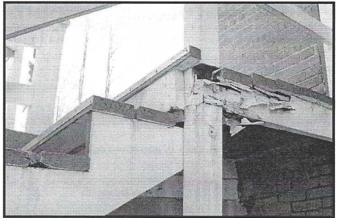
Repairing the stairs to the lower level yard was on the top of list of repairs to make this past summer.
